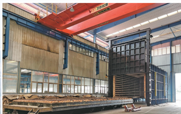
机身壁炉回火 Machine frame annealed in electrical grate
